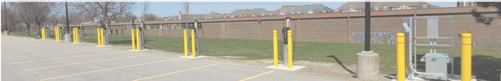
The picture is a charging station designed, installed, and commissioned by Signature Electric for a pharmaceutical client in North York
